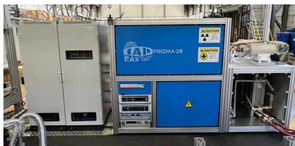
Fig. 2. Photograph of the 28 GHz / 10 kW-based complex for ion sources in JINR
